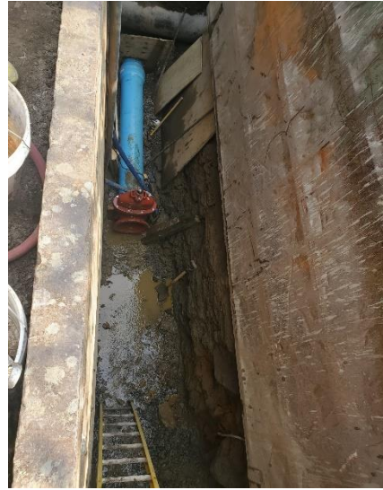
Photo 2: Installation of Force Main 12'' PVC Drain Lines at the Auburn Street Pump Station
