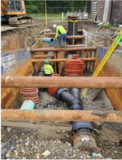
Photo 1: Installation of Launching Barrel and Associated Pipe and Fittings for Force Main Tie-in Connection at the Auburn Street Pump Station
