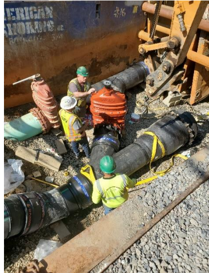
Photo 4: Installation of Fittings for Force Main Tie-in Connection at the Auburn Street Pump Station
