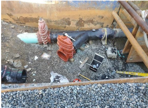
Photo 3: Installation of 20" Gate Valve for Force Main Tie-in Connection at the Auburn Street Pump Station
