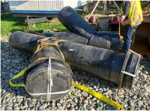
Photo 1: Revised Fittings for the Auburn Street Pump Station Force Main Tie-in Connection
