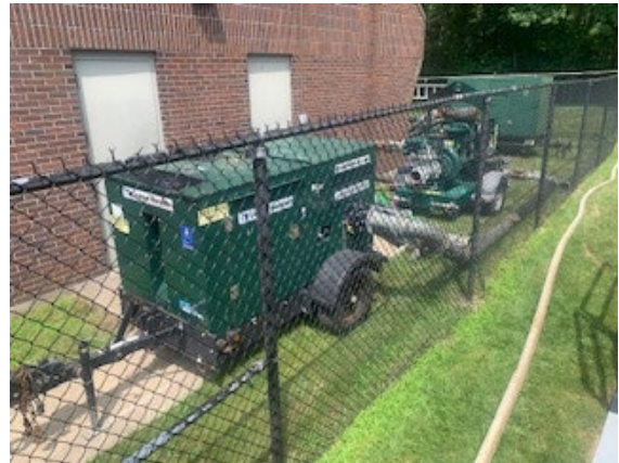
Photo 4: Bypass Pumps at Auburn Street Pump Station
