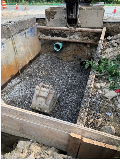
Photo 1: Exposure of 20-Inch PVC Force Main
