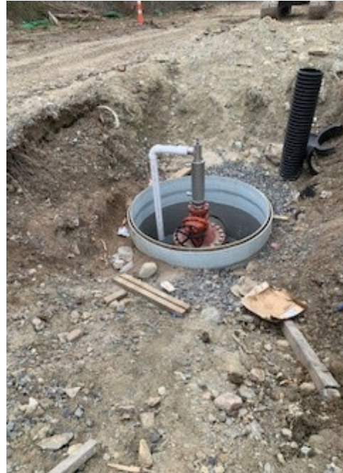
Photo 2: Air Release Valve with 3" PVC Discharge Pipe
