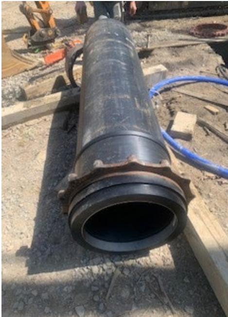
Photo 1: HDPE Pipe with Fused PVC Transition
