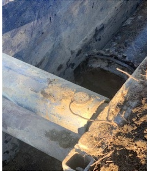
Photo 1: HDPE Sewer Force Main Installation Capped at end of Thatcher Street for Testing
