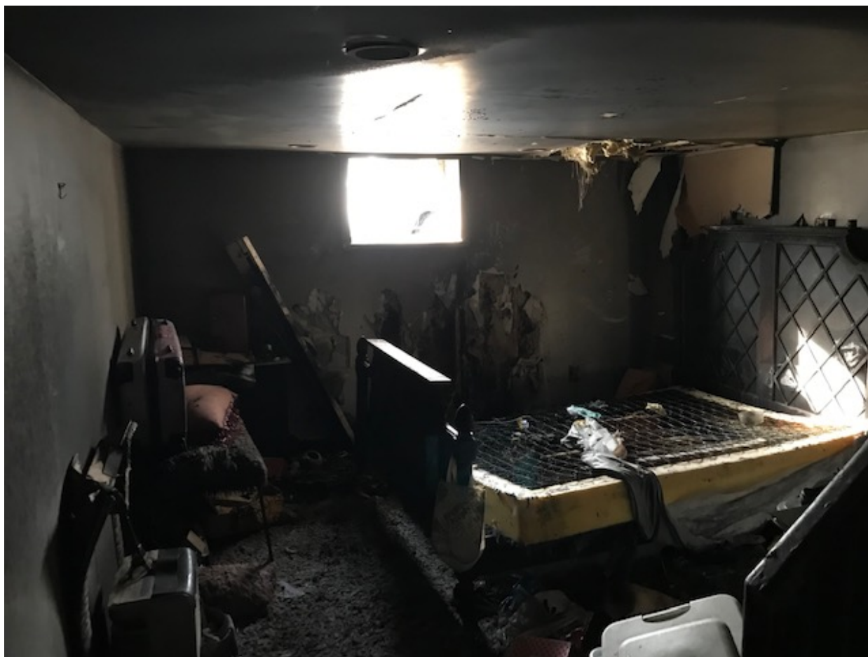
The basement of a School Street home in Whitman sustained heavy damage during a fire Wednesday, Jan. 8. (Photo courtesy Whitman Fire Department)
